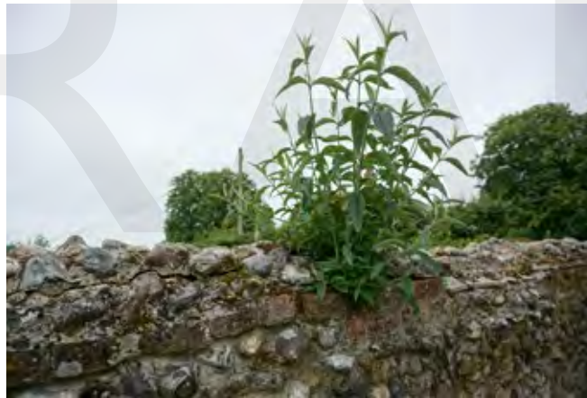
Vegetation growth on historic walls in the churchyard
