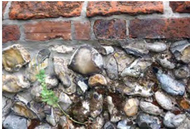
Cement pointing to an historic wall
