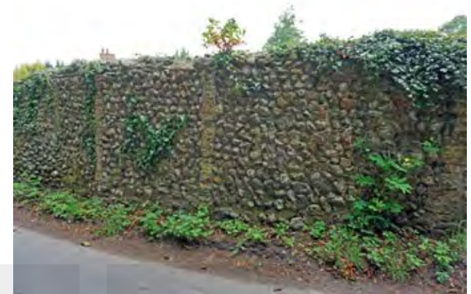
Vegetation growth on historic wall to the churchyard
